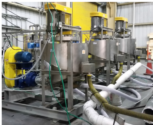
Fig. 6. Feed sump/pump arrangement and three-stage StackCell™ test circuit.
